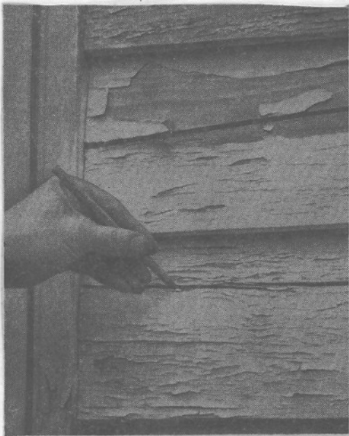
Rot is beginning to set in in some of the project's siding.
